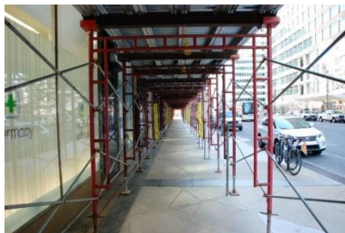
Safety canopy above walkway
